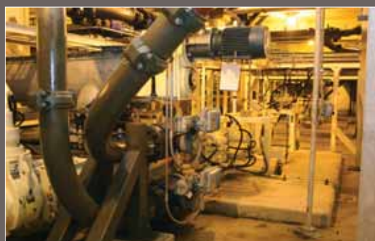
The pumps in place at YCUA continually move cake, which has been increased in solids content from 3% to as much as 25%.
