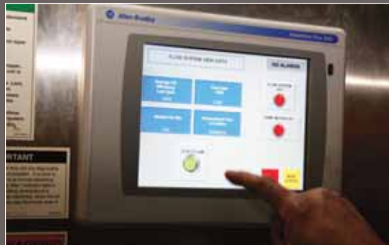
Ypsilanti plant managers have accommodated double-digit population growth and now can handle peak flows to 72 mgd.
