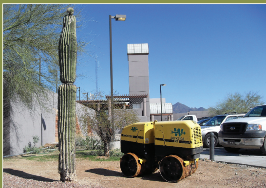
Significant population growth combined with a limited water supply signaled to Scottsdale plant managers that an upgrade was needed.
