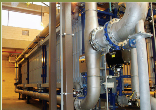
The Siemens CP MF membrane system installed at the CAP plant is the first and largest in the U.S.
