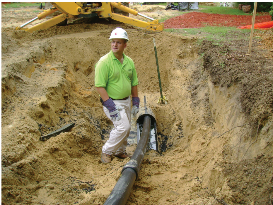
Pete Monday, a Geospatial employee, at the Oak Island, N.C., site. A pipeline mapping system provided the town with plan and profile reports, as-built drawings and positional data for a vacuum sewer system installation.
