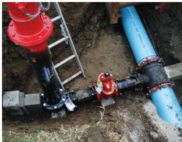
The town of Celina’s new water lines would not integrate well with existing infrastructure—decades-old rusty ductile iron pipe ready to rupture.
