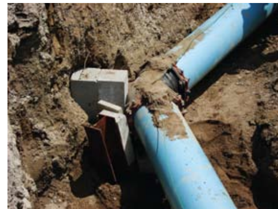
Plastic pipe eases worry about rusting, which consumes the chlorine residual that kills fungal growth in a water system, and “red water” complaints from customers.
