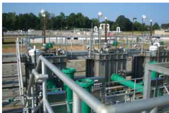
Other plant equipment forms a backdrop for one part of the filter lineup.
