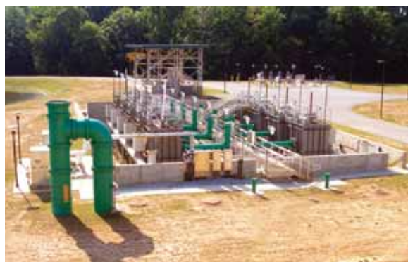
A view of the complete filter basin.
