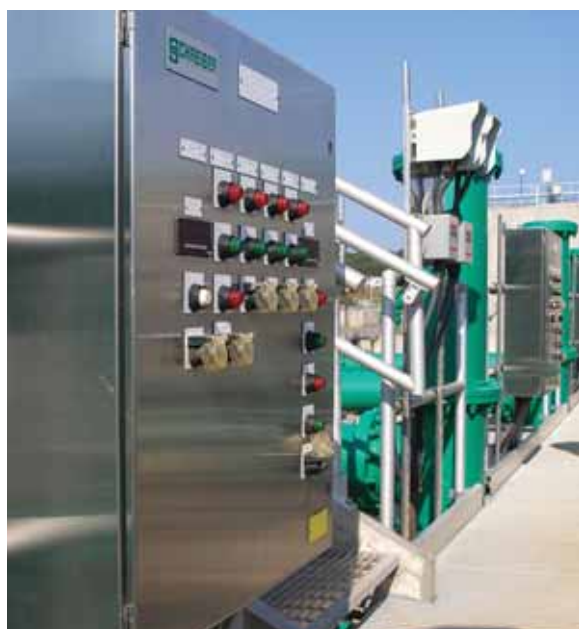
One of nine control panels; there is one for each filter position.
