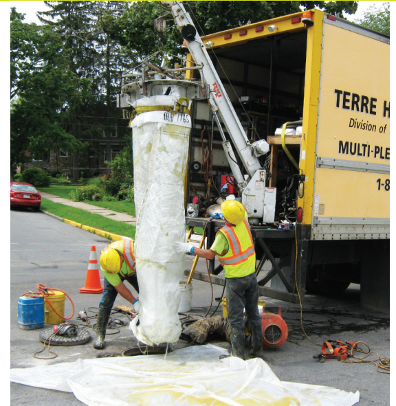
PPM installed Lightstream technology, a UV light-cured fiberglass CIPP lining, in the sanitary sewer mains.
