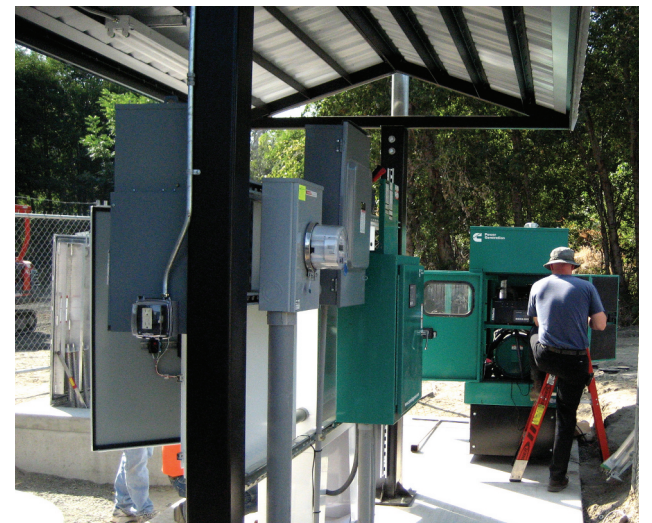
The city received a pre-engineered package lift station as part of a package deal, saving a lot of time.
