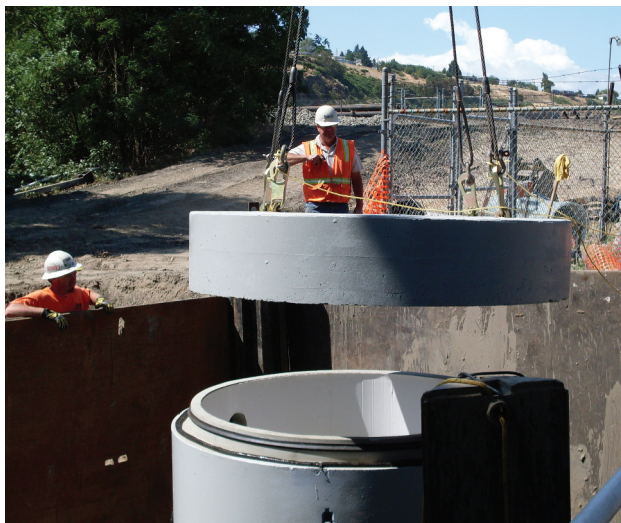
Features of the new pump station include an emergency generator, onsite control interface and interior lining of the wet well.
