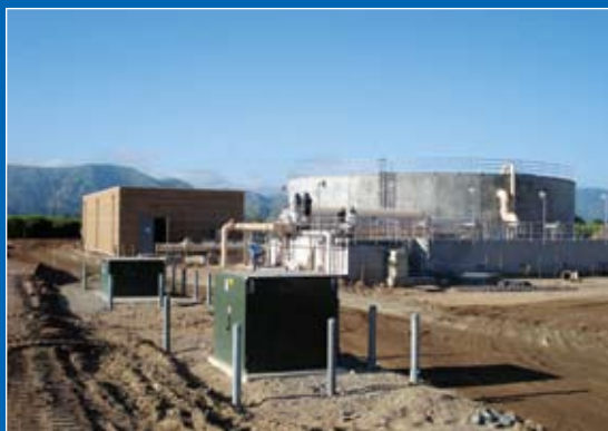
The water recycling facility emits no discharge into the Santa Clara River and reuses 100% of its effluent—a rare attribute of coastal water plants.
