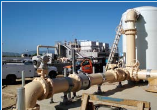
Approximately 200,000 gpd of reclaimed water is used for irrigating city parks and green areas throughout the city of Fillmore.
