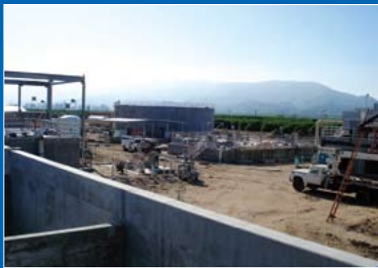
The plant currently treats about 1 mgd, but can be upgraded to 2.4 mgd in the future.
