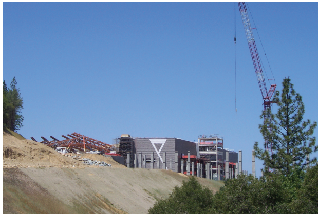
Red Hawk Casino was designed to treat and dispose of all its wastewater on site.
