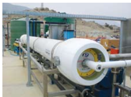
Pilot plant using new RO elements.
