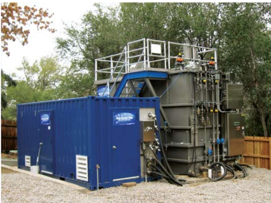
Aqua-Aerobic MBR system at Colorado School of Mines.
