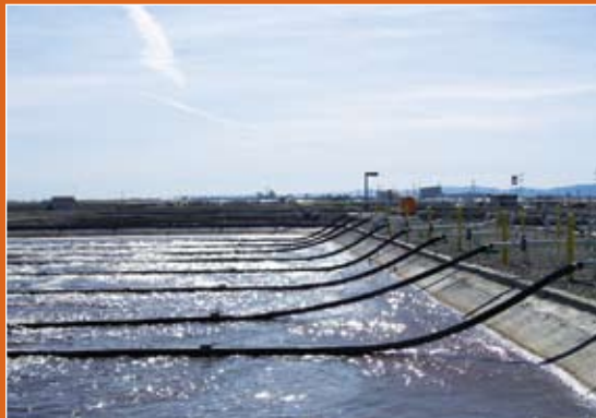
The Willows WWTP extends across 26 acres, comprises 24 miles of mainlines and includes five lift stations.
