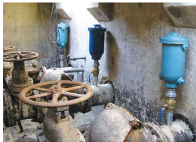
Each valve is installed on a raw sewage main, and the mains run parallel in the vault.
