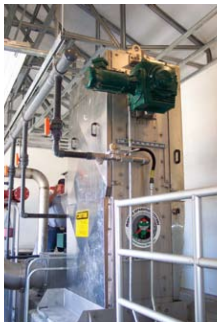
The new separation system provides initial solids screening, protecting the MBR and eliminating aerator plugging.
