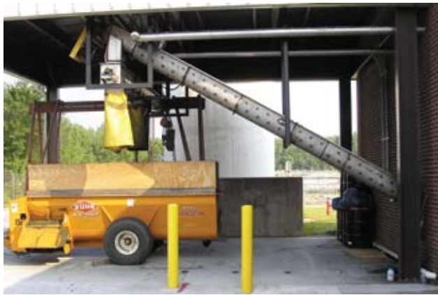
A biosolids drying system was retrofitted into the existing space in Farmville.
