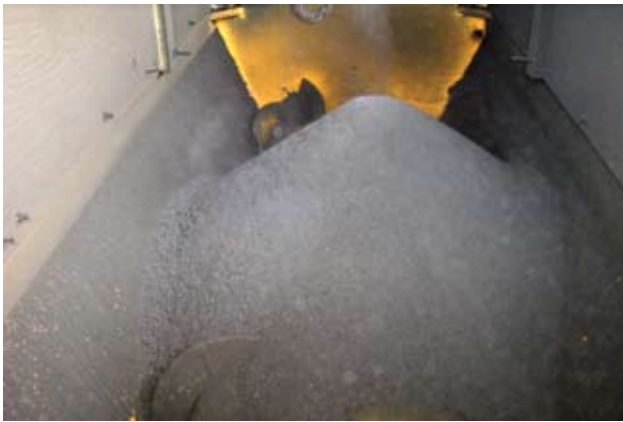
Due to off-peak electricity restrictions, operating personnel are required to adjust what time of day they run the dryer based on the time of year.
