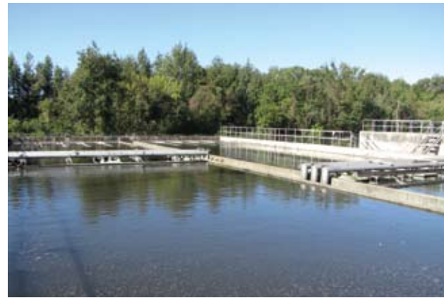
The new system was up and running in September 2007 and now produces Class A biosolids.
