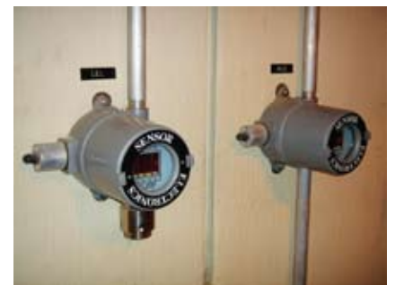
Detectors in a long underground tunnel beneath the clarifier/aeration basins keep constant watch for toxic/explosive gas buildup. Digital readout panels show actual gas levels; LEDs glow green if levels are normal and change to amber then red if readings increase.
