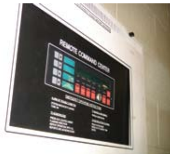
Three remote command centers monitor the army of gas detectors and flash immediate warning of trouble conditions anywhere in the treatment facility. Systems also check every detector every 5 seconds, reporting any problems instantly.
