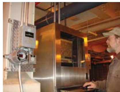
Scattered throughout the plant, sensitive detectors show actual gas levels in ppm or LEL. A cubicle panel shows plant pumps/valves schematic.
