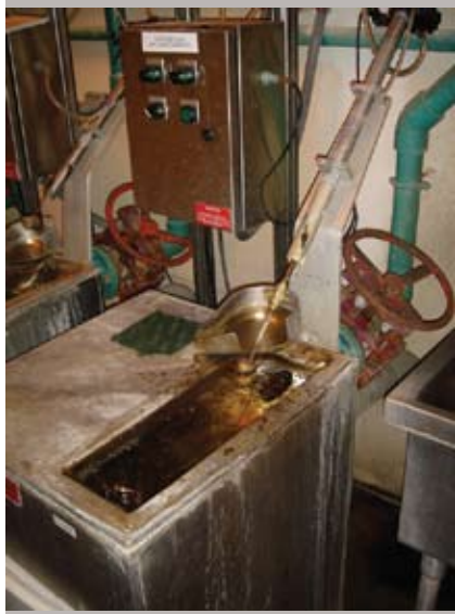
A tiny bucket scoops up a sample of water leaving the Seneca WWTP before it flushes into the nearby Minnesota River. Samples are tested for cleanliness and clarity, and discharge is purer than upstream river water.
