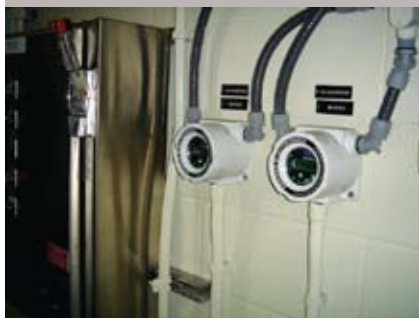
Twin detectors monitor chlorine (Cl 2 ) and sulfur dioxide (SO 2 ) levels in the tank feed room. Because chlorine is heavier than air, sensing tubes go down to floor level. Besides watching for chlorine, detectors watch themselves, reporting problems on a digital readout panel, relaying an alarm to a remote command center.
