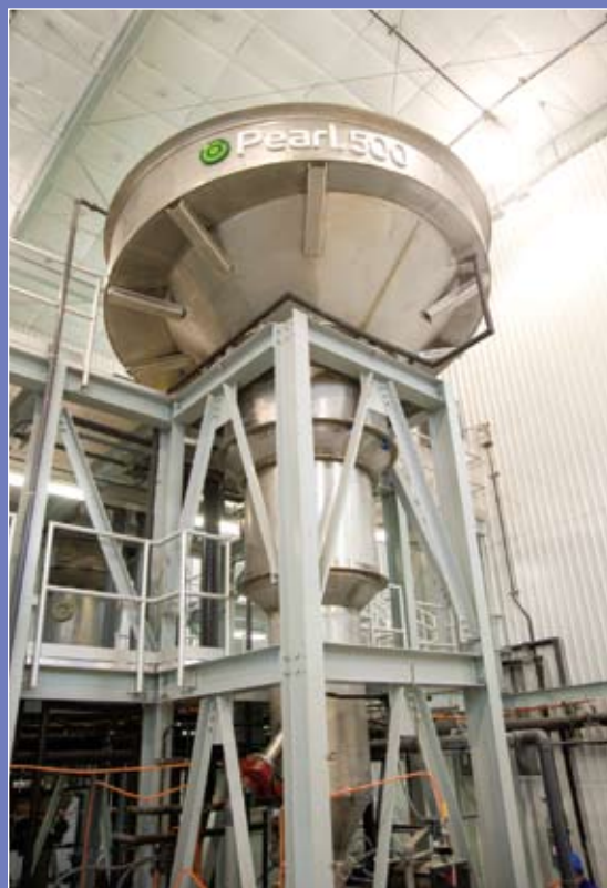
Three reactors installed in the facility have the ability to recover 1.5 tons of fertilizer on a daily basis.
