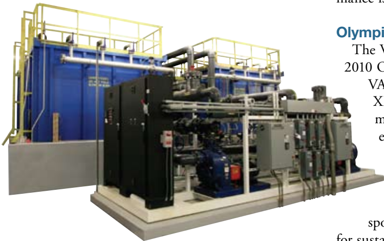
VCC's onsite wastewater treatment system combines an activated sludge process with UF membranes.
