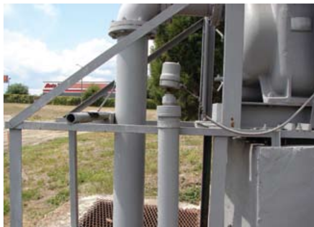
Zephyrhills municipal public works staff was relieved when the new sensor and pump control system performed effectively in a flash flood just weeks after installation.
