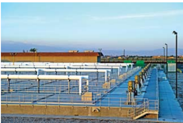
Covered aeration basins achieve the zero-odor plant goal.
