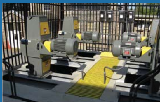
Rapid-mix and flocculation basins send water to membrane trains.
