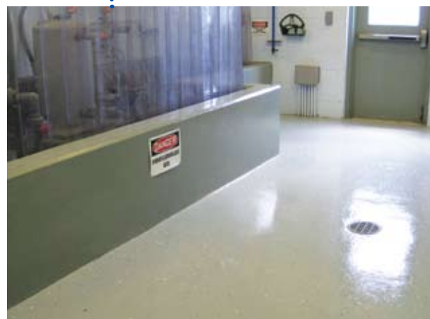
In the Cooper City facility, floor coating was installed in the plant's membrane building.
