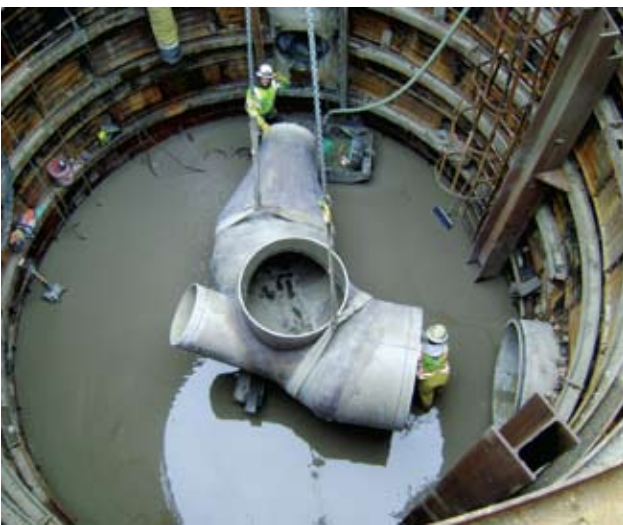
Design of the Trunk Interceptor Project was based on the Marysville Wastewater Master Plan.
