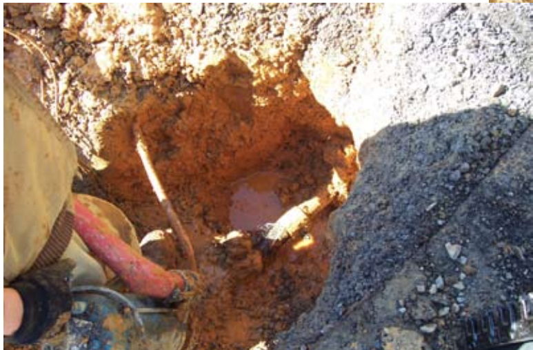
The city worked with Johnson Controls to diminish its real and apparent water losses.
