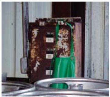
A metal enclosure exposed to heavy moisture in the Abita Brewery facility in Louisiana had to be replaced sooner than anticipated.
