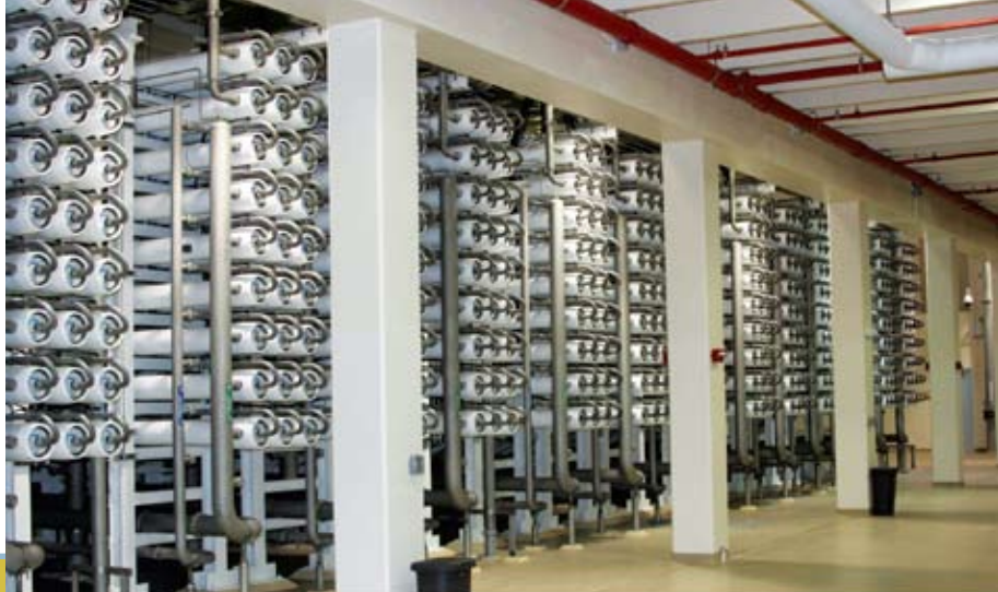
The membrane hall. Array is 63:18 with second stage at the top.
