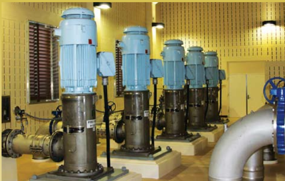
NF feed pump room, with cartridge filter discharge to the right.
