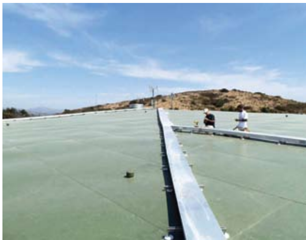
The cable/cable tray holding system set the OMWD rehabilitative painting project back on track.
