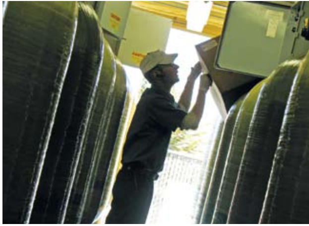
The multi-bed, PLC-controlled treatment systems use 16 or more resin vessels depending on flow rates.
