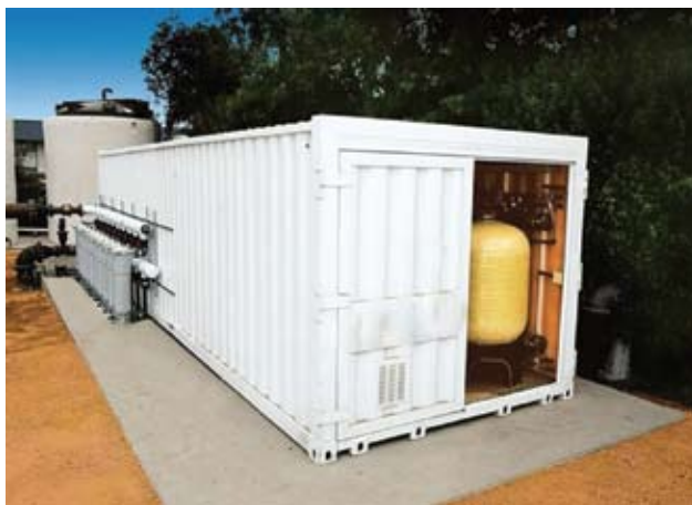
All of the Envirogen systems at Cal Water Salinas sites feature a 10-year services agreement that guarantees performance for the life of the asset, volume of salt consumption, volume of waste brine and finished water quality. The agreement covers all treatment equipment and associated connections.
