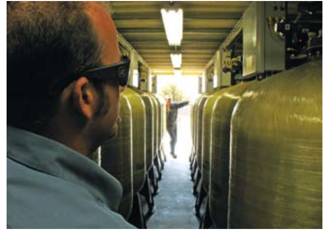
In order to run efficiently at the lowest possible operating cost, treatment systems at Cal Water Services sites are monitored and adjusted continually.
