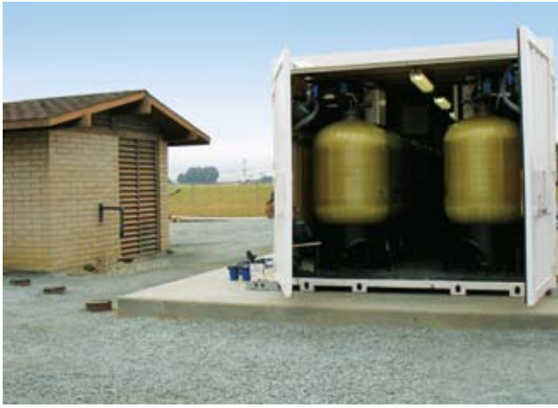
The ion-exchange systems for nitrate removal are mobile and containerized for rapid deployment and offer a small footprint for space-challenged drinking water utilities.
