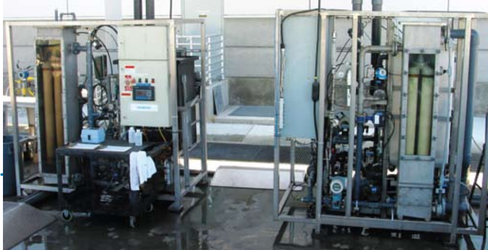
CS pilot systems at the GWRS pilot-plant facility
