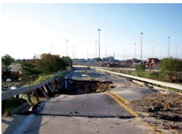
Damage caused to a roadway by a 72-in. water main break in Baltimore.
