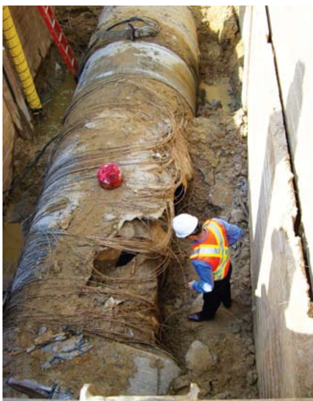
Inspection of a 72-in. water main break in Baltimore.
