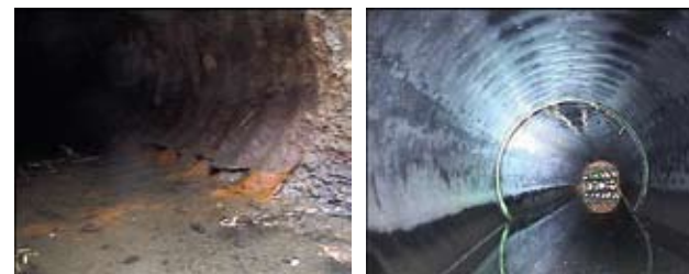
Left: Steel pipe is susceptible to corrosion from saltwater. Right: An inspection photo showed no signs of soil migration through the joints or visual deflection of the pipe.
