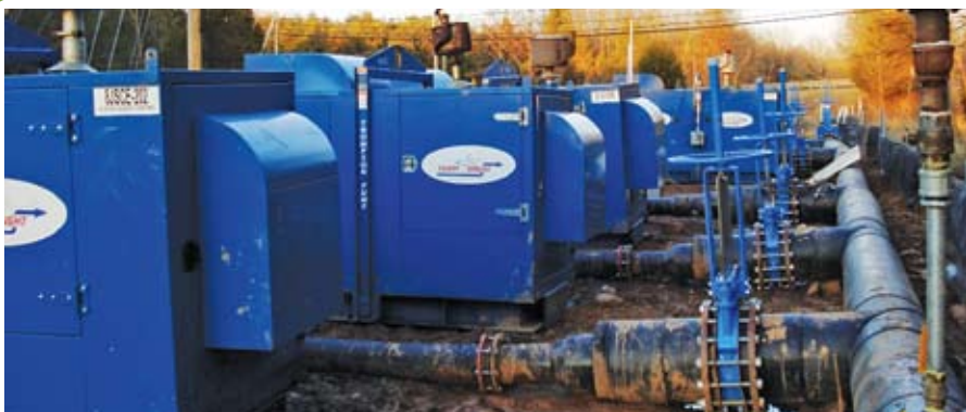
Centerville, Va., ultimately hopes to replace more than 5 miles of pipe. Bypass systems diverted flows around pipe sections being replaced.
