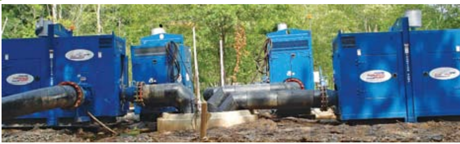
Each of the project's 10 core bypass phases includes a main bypass and multiple lateral bypass tie-ins.
