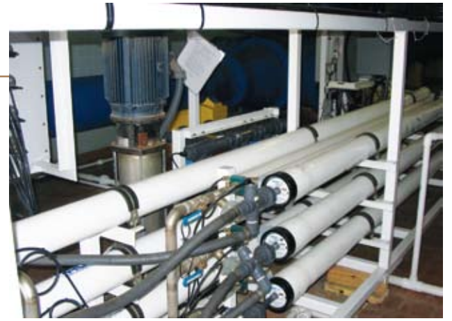
Retrofitting existing multimedia filters with ultrafiltration proved to be a beneficial decision for Manatee County.
