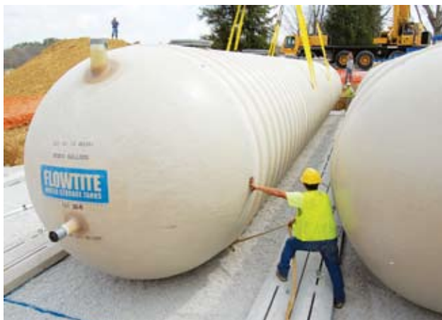
The Lexington Sanitary Sewer Project entailed the installation of a 10,000-gpd communal system.
