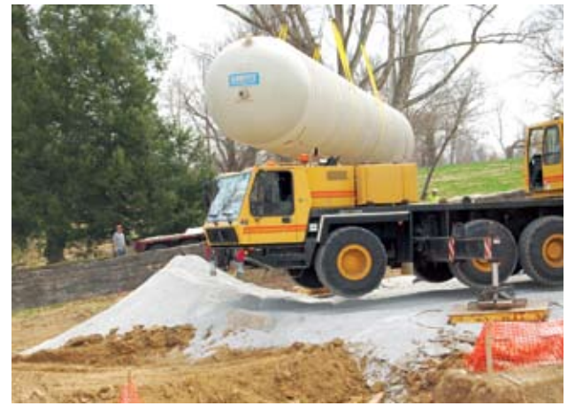
Rural communities often struggle to afford conventional wastewater collection and treatment methods.
