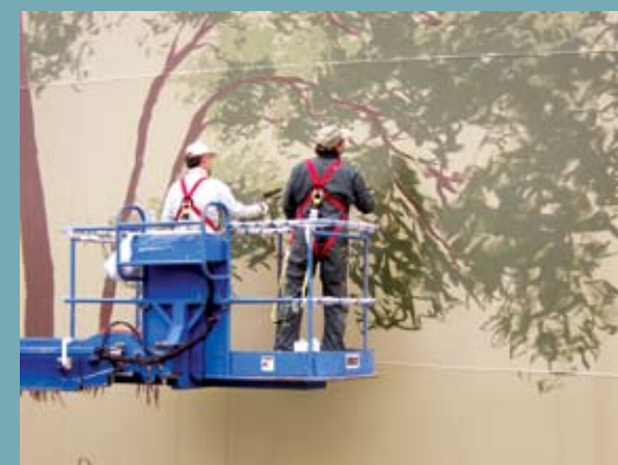
The Goetzingers use a boom lift to reach all parts of a tank. They paint the top if nearby buildings are taller than the tank.
