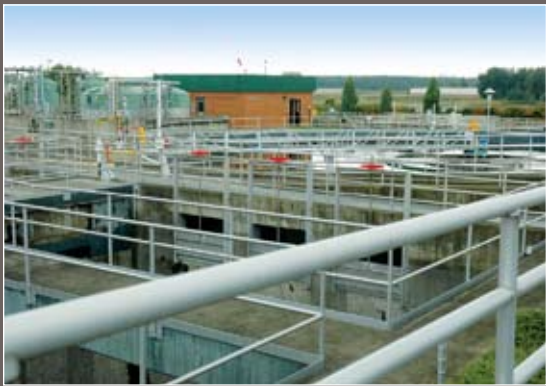
Gresham WWTP serves more than 100,000 customers, with flows averaging about 13 mgd.
