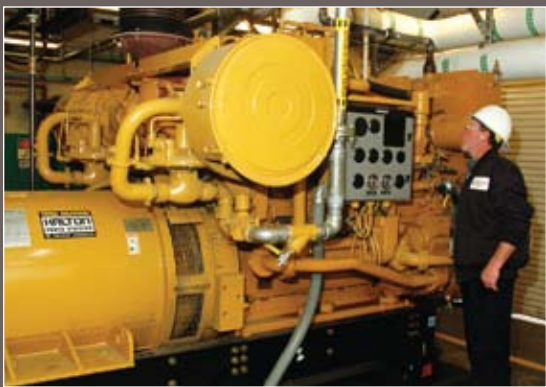
A cogeneration engine converts the plant's digester gas into energy for electrical power and heat.
