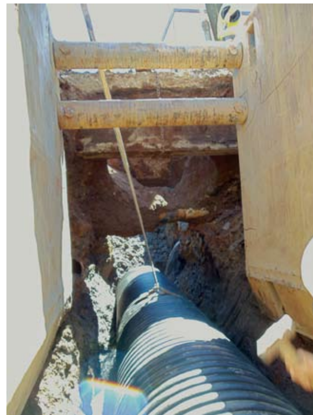
Using HDPE pipe solved a number of challenges associated with this project.
