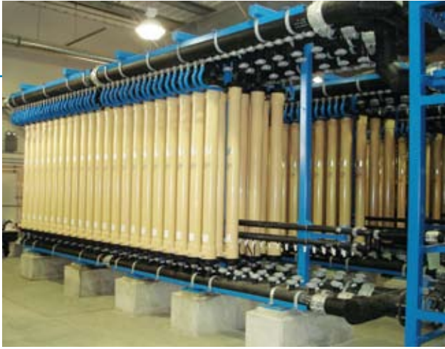
The custom MF system at West Elgin, Ontario, Canada, uses high-crystalline PVDF membranes.
