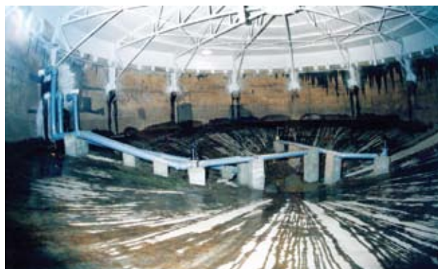
Inside the JetMix installation at the Wheaton WWTP.
