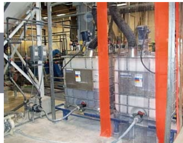
Acid is automatically pumped into the batch tank to shock the pH and separate the solids. Lime is used to precipitate the metals and neutralize the water.
