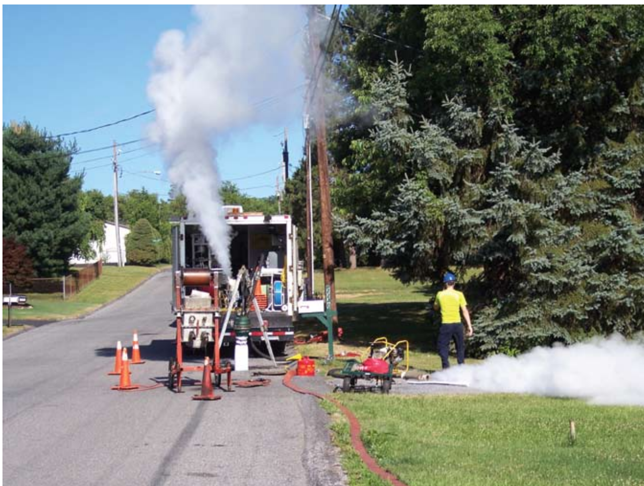
Cleanouts included a storm sewer casing backfilled with select material and a cast-iron frame to prevent future damage.
