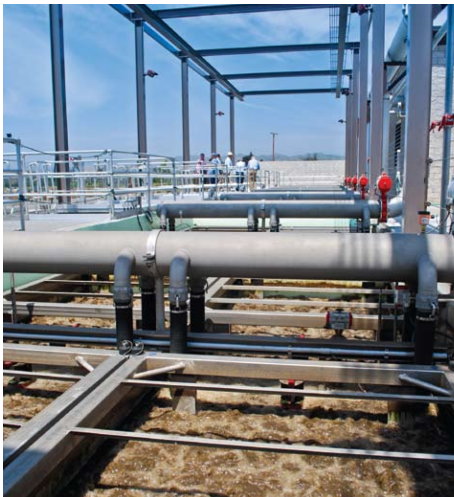
The new MBR facility is designed to handle a 7.2-mgd peak daily flow.
