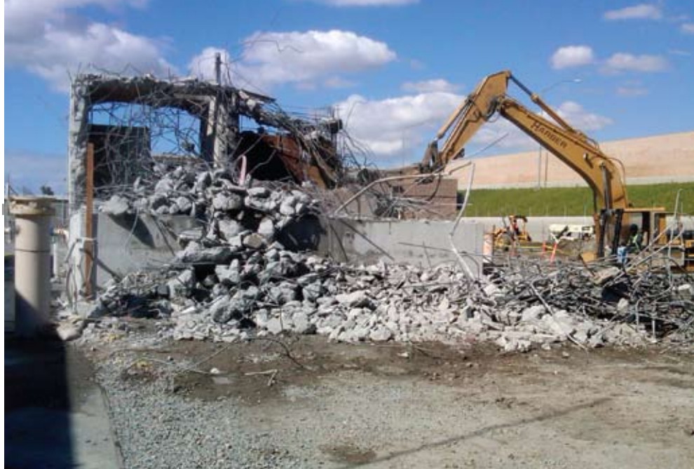
The existing ozone contactor will be converted to a transfer pump station.
