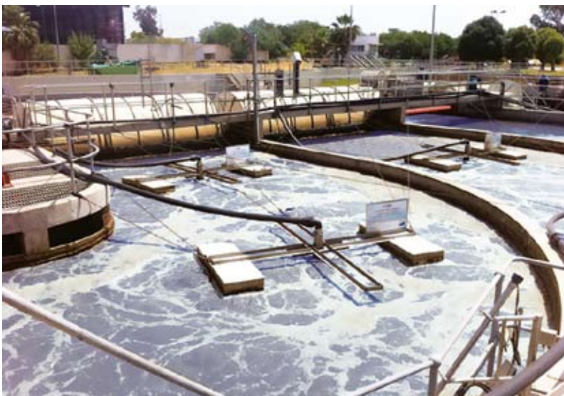
Fine-bubble aeration systems reduced the plant’s energy consumption by about 55% and improved odor control.
