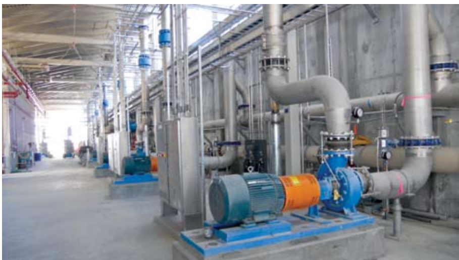
The City of North Las Vegas Water Reclamation Facility, with the largest operating MBR in North America, will provide reclaimed water for use in industrial and recreational applications.
