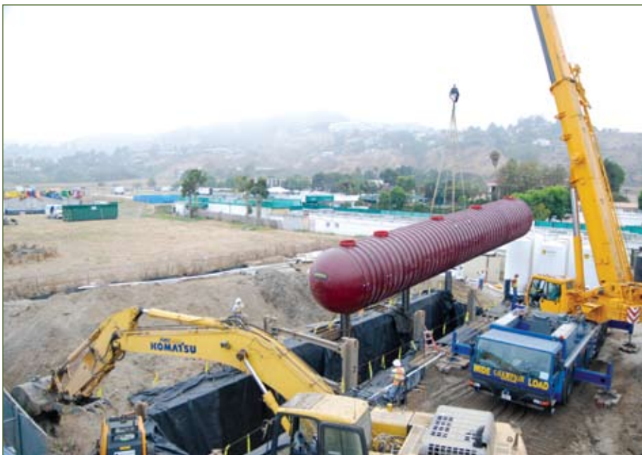
Installing the 75-ft MBR system tank through the shoring structure. (Photo courtesy of Integrated Water Services Inc.)
