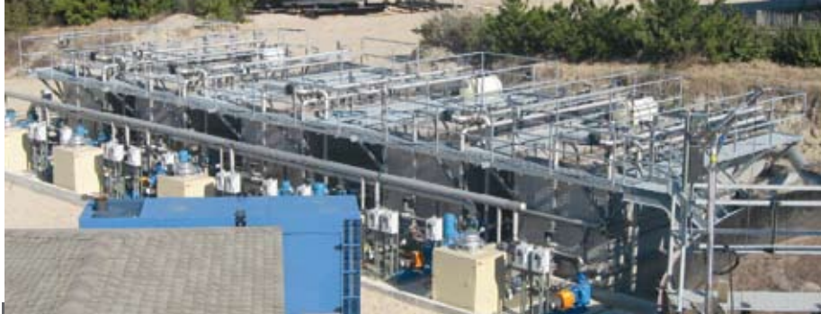
Population growth drove the need for additional capacity and capabilities at the Monterey Shores WWTP.
