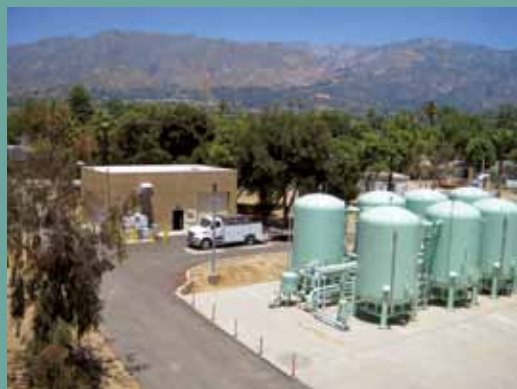
Treatment tanks use ion exchange to remove perchlorate from groundwater, meeting state maximum contaminant level regulations.
