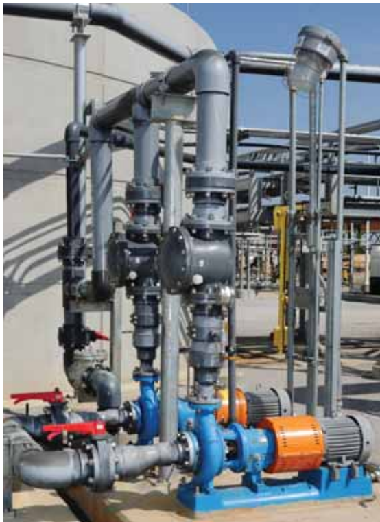
The plant was built with operability in mind, with operations and maintenance teams participating in design reviews.
