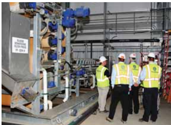
The facility's multifaceted wastewater treatment system consists of three separate treatment systems.
