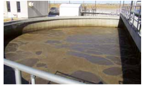
HYBAS system retrofitted into a circular basin at Dry Creek Wastewater Treatment Plant in Cheyenne, Wyo.
